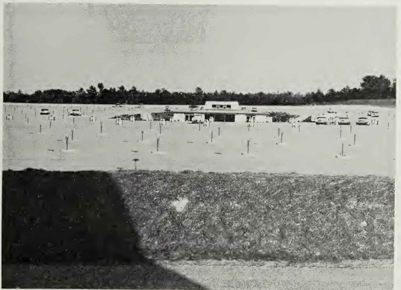
Large units visible at speaker post sites are for combination heat-air conditioning. Presently, facilities for the Carrier units can handle 80 cars. Weiss plans to expand the service if the demand for the air-conditioners/heaters is great enough.
